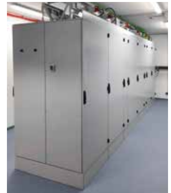
Rear view of the IS-1 racks with cable tray and outlet boxes at the top.
