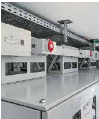
Overhead cable trays with outgoing boxes and busbars.
