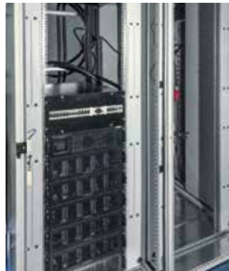
Technology rack in the construction phase with UPS system and battery pack from SCHÄFER IT-Systems.
