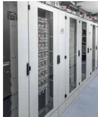
IS-1 four-cabinet system with redundant, in-line SideCoolers CW.
