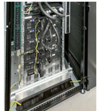
Rear view of the technical rack with on-site supply cable, outlets to the busbars and SCHÄFER Smart PDUs.
