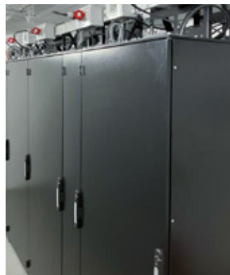
Rear view of the IS-1 racks with cable tray and outlet boxes at the top.
