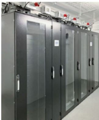
IS-1 Edge Row Type 4 four-cabinet system with two SideCoolers from SCHÄFER IT-Systems mounted in a row.
