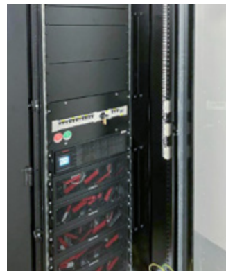
The centrepiece of the system: Technology rack with Powerbox and UPS system from SCHÄFER IT-Systems.
